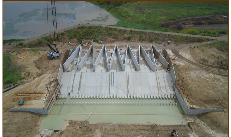
Aerial view of the site 6 Dam rehabilitation project showing the labyrinth weir spillway
