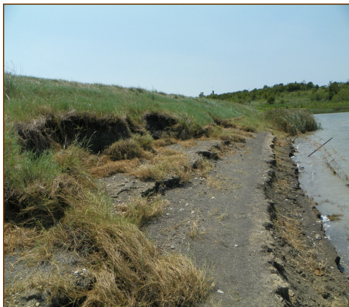
Significant erosional damage along the face of the upstream embankment for Site 10 following the 2017 flooding.
