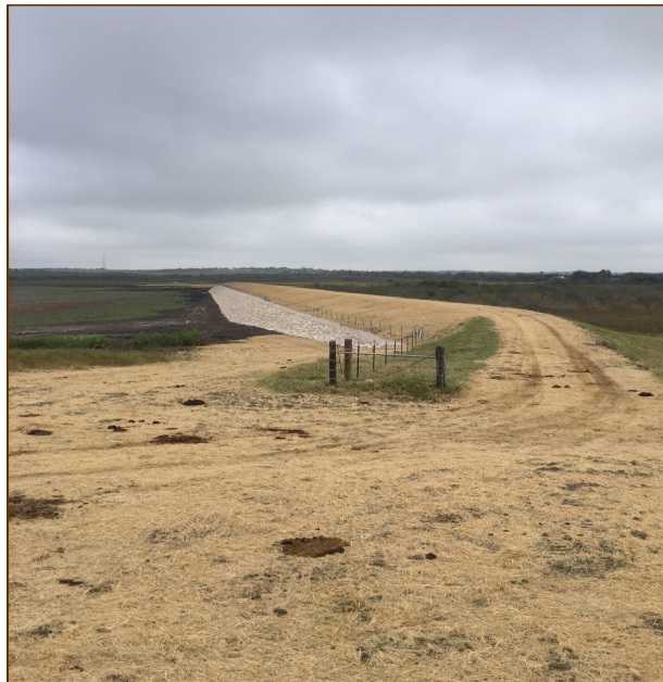
Site 12 EWP completed construction looking at the upstream embankment with installed riprap
