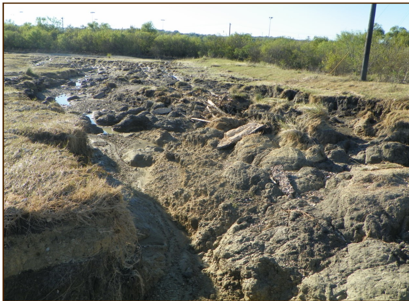
Site # 6 Flood Damage to Auxiliary Spillway
