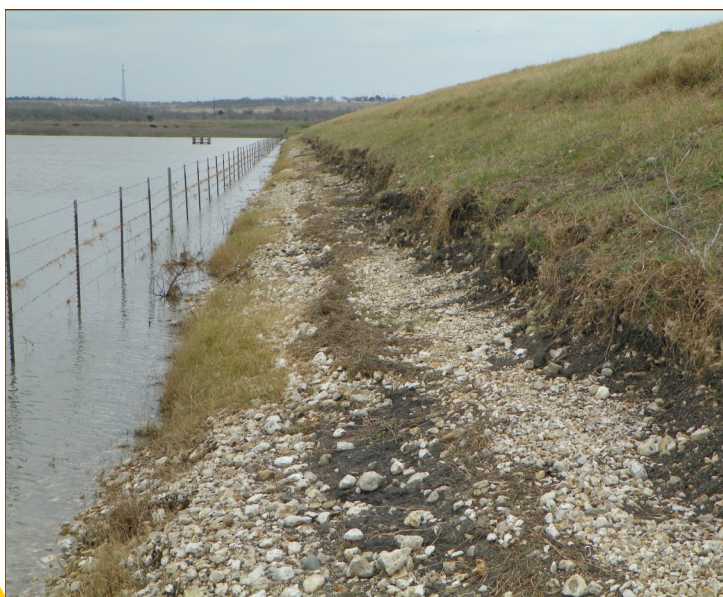
Significant erosional damage along the face of the upstream embankment for Site 12 following the 2015 flood.
