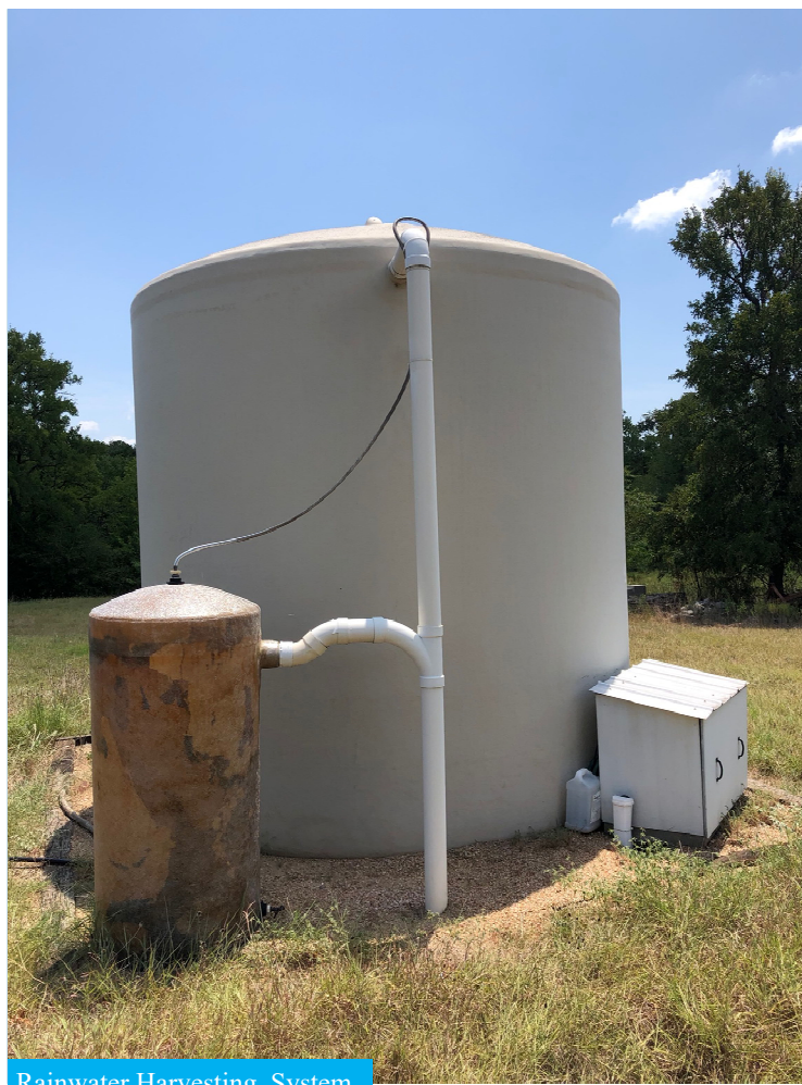
Rainwater Harvesting System
